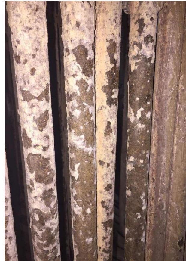
Water pipe corrosion thinning
